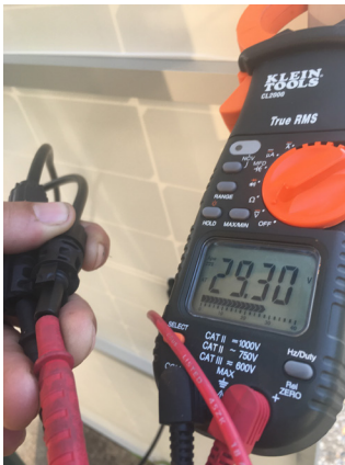
6. Module Voc multimeter measurement
